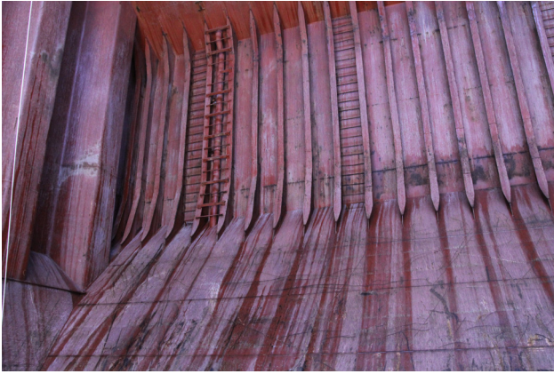
Figure 1. Damaged paint coating showing white stains and chalking, typically encountered when sodium hypochlorite is used. In addition, black rust is seen, under-rusting the coating. The only remedy is paint maintenance.
